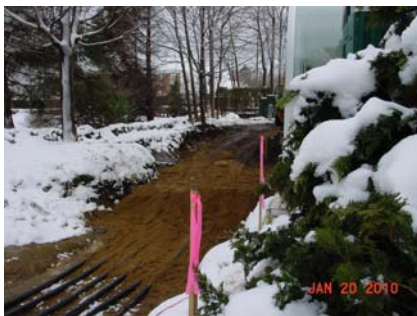
Header pipes run to mechanical room from borehole field
