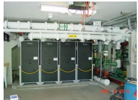
Water-to-water ground source heat pumps were installed, with total heating capacity over 140 tons.
