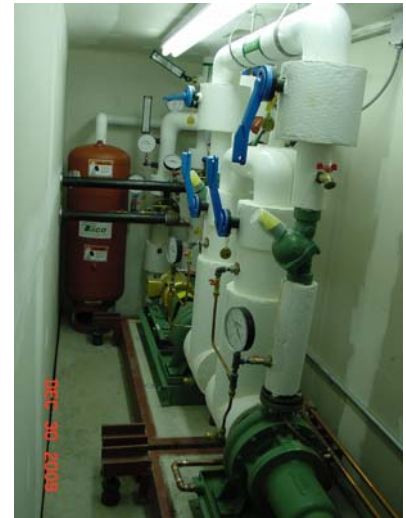
Variable speed ground loop pumps were used to conserve pump energy.
