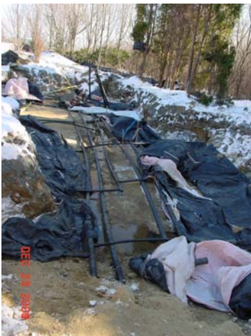
13 boreholes were drilled. Boreholes were ganged together to form a ground loop system. Header pipes of the ground loop run to the pump room inside the house.
