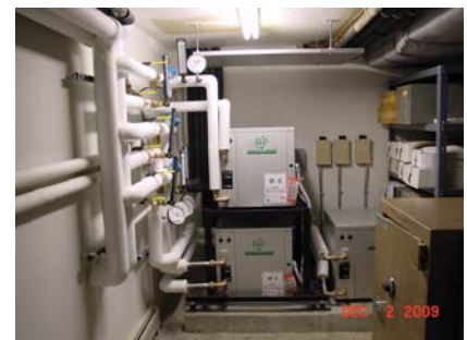
Ground source heat pumps were installed in mechanical space inside the house
