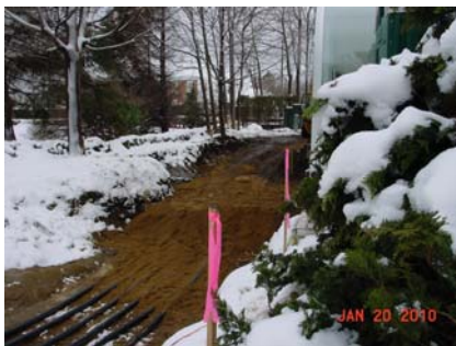
Header pipes run to mechanical room from borehole field
