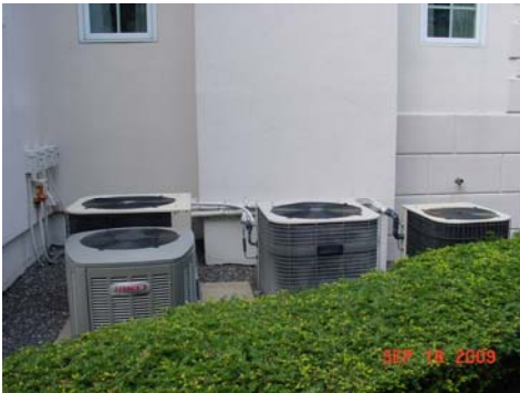
The 6 existing outdoor condensing units were no longer needed and were removed.
