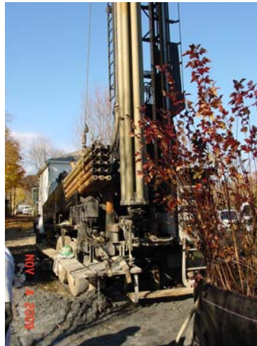
Compressed air rotary DTH hammer drill rig was used to drill the vertical boreholes.
